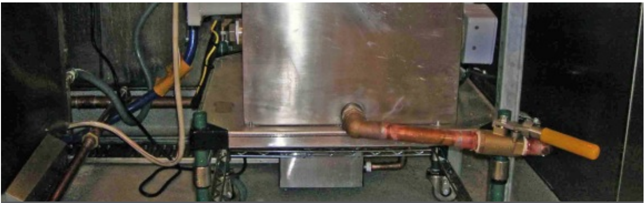
Front of Goslyn with silt valve plumbed using street elbow
