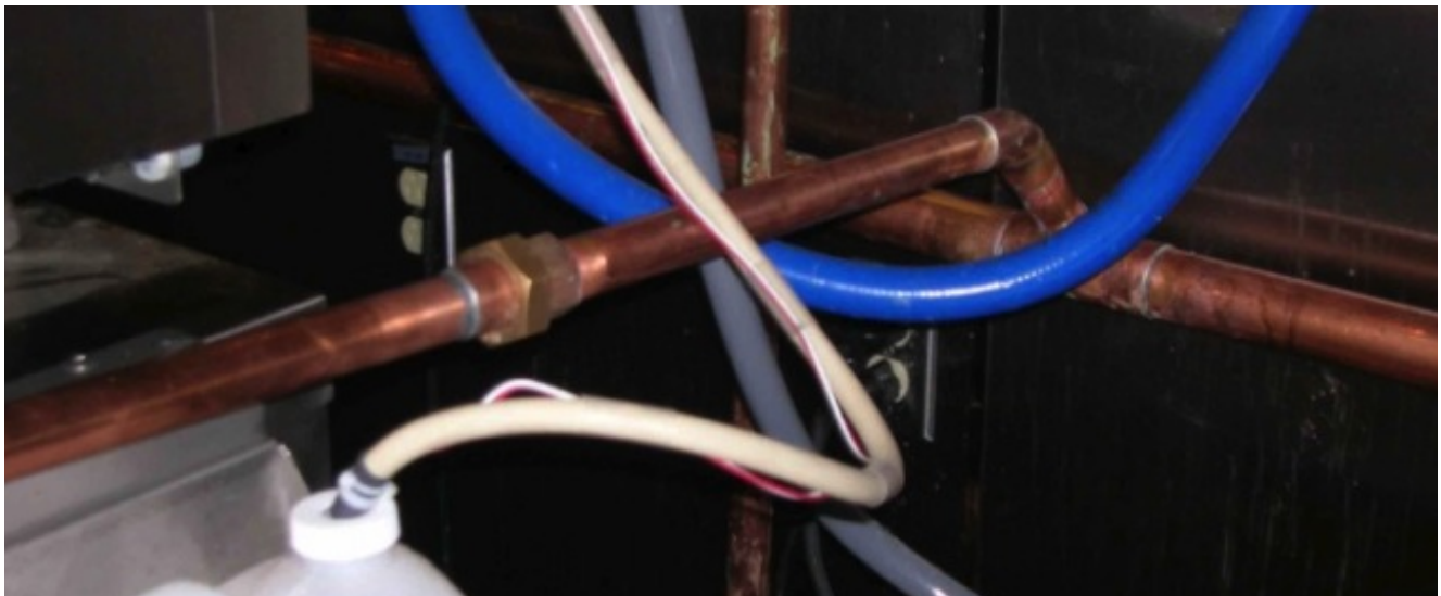
Plumbing shown from the 2nd Top Rotisserie Oven connected to the drain from the 1st Top Rotisserie Oven
